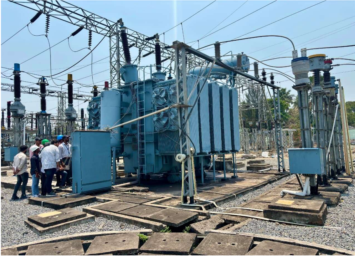
40 MVA TRANSFORMER (132/33 KV)
