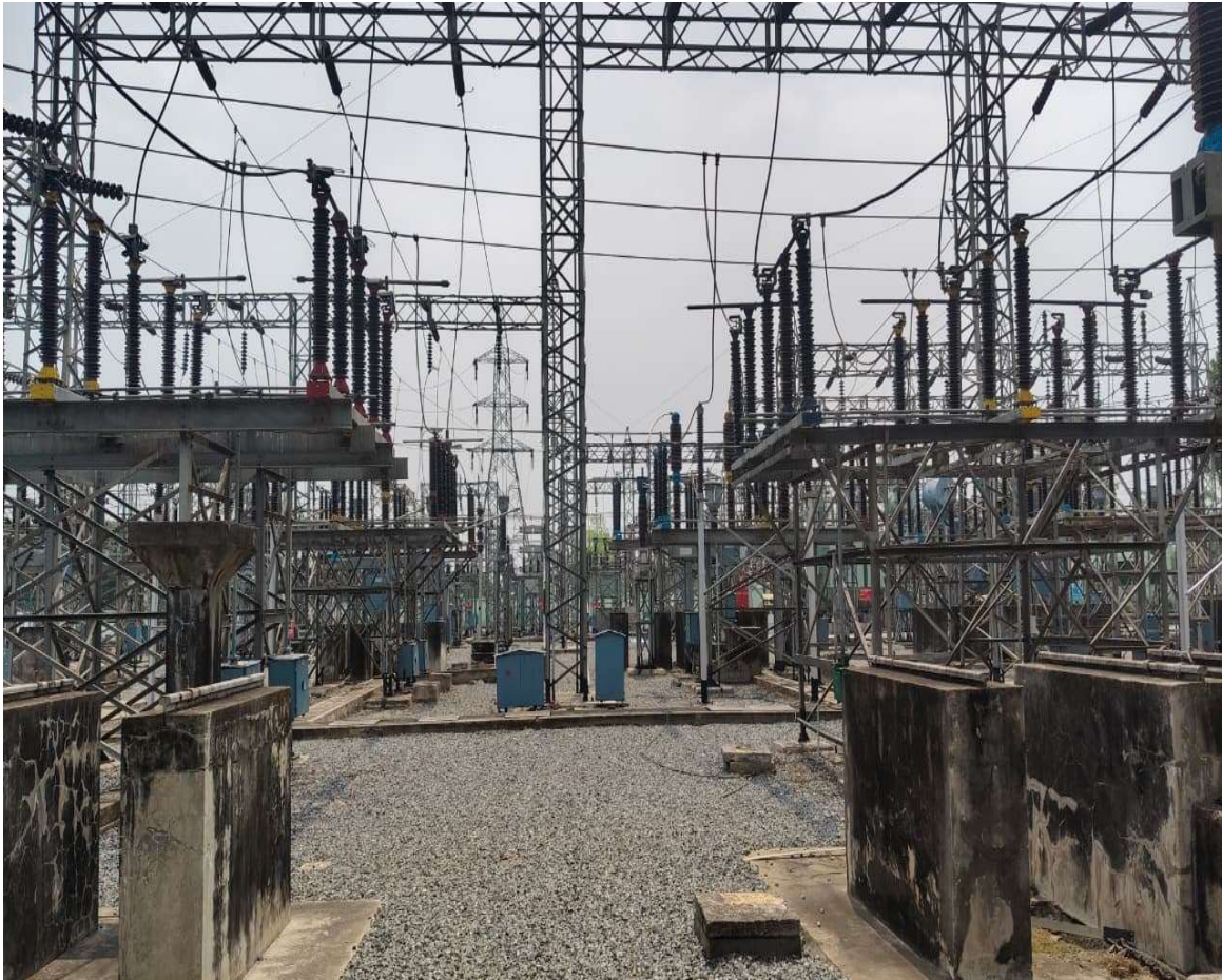
POWER GRID OF OPTCL, AMBAGADA, BRAHMAPUR
